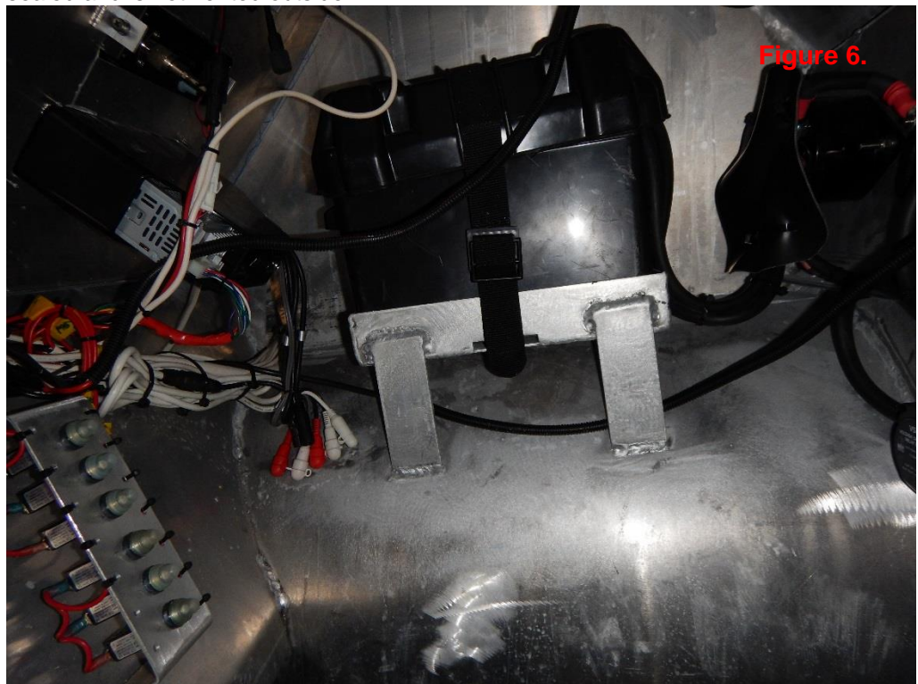
Figure 6. Batteries are to be in a location away from sources of ignition. Battery box is not sealed and is not vented outside.
